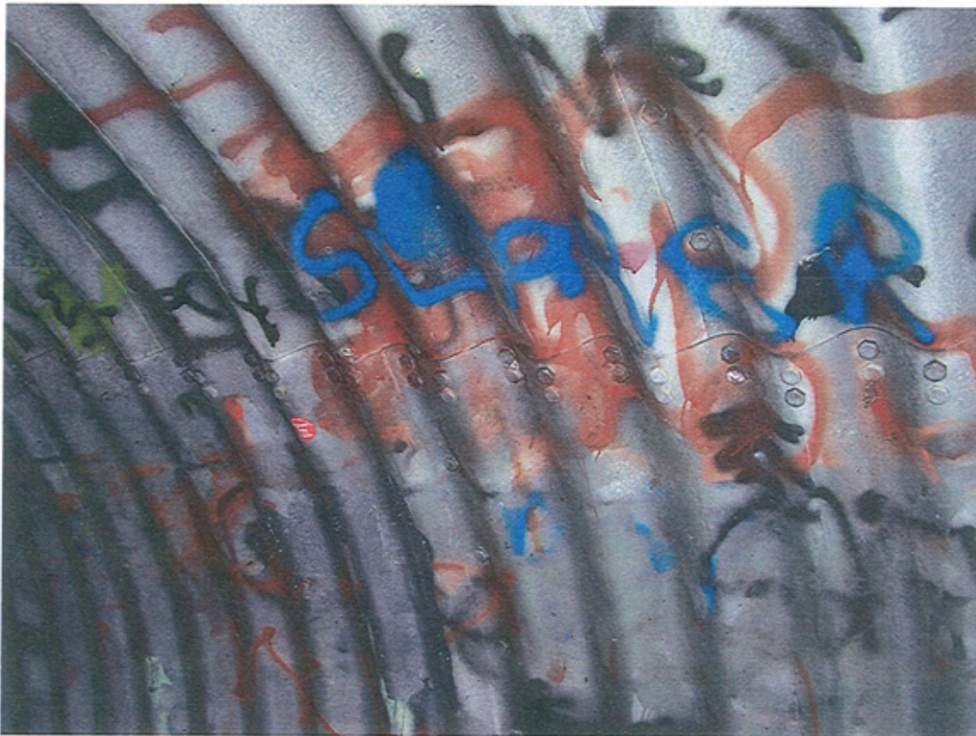
An example of graffiti on the tunnel walls
