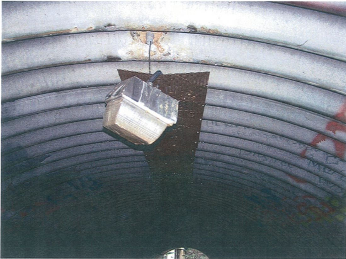
An example of a broken lighting fixture
