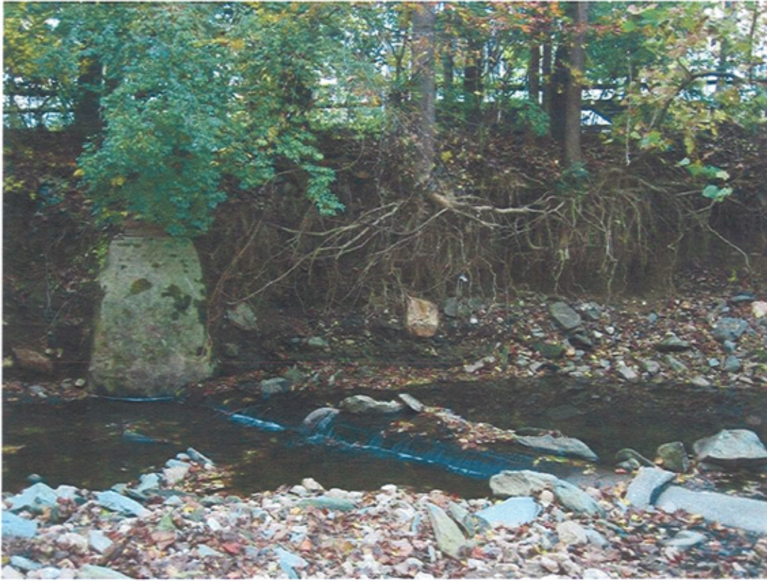
Sewer line and manhole structure exposed by erosion.
