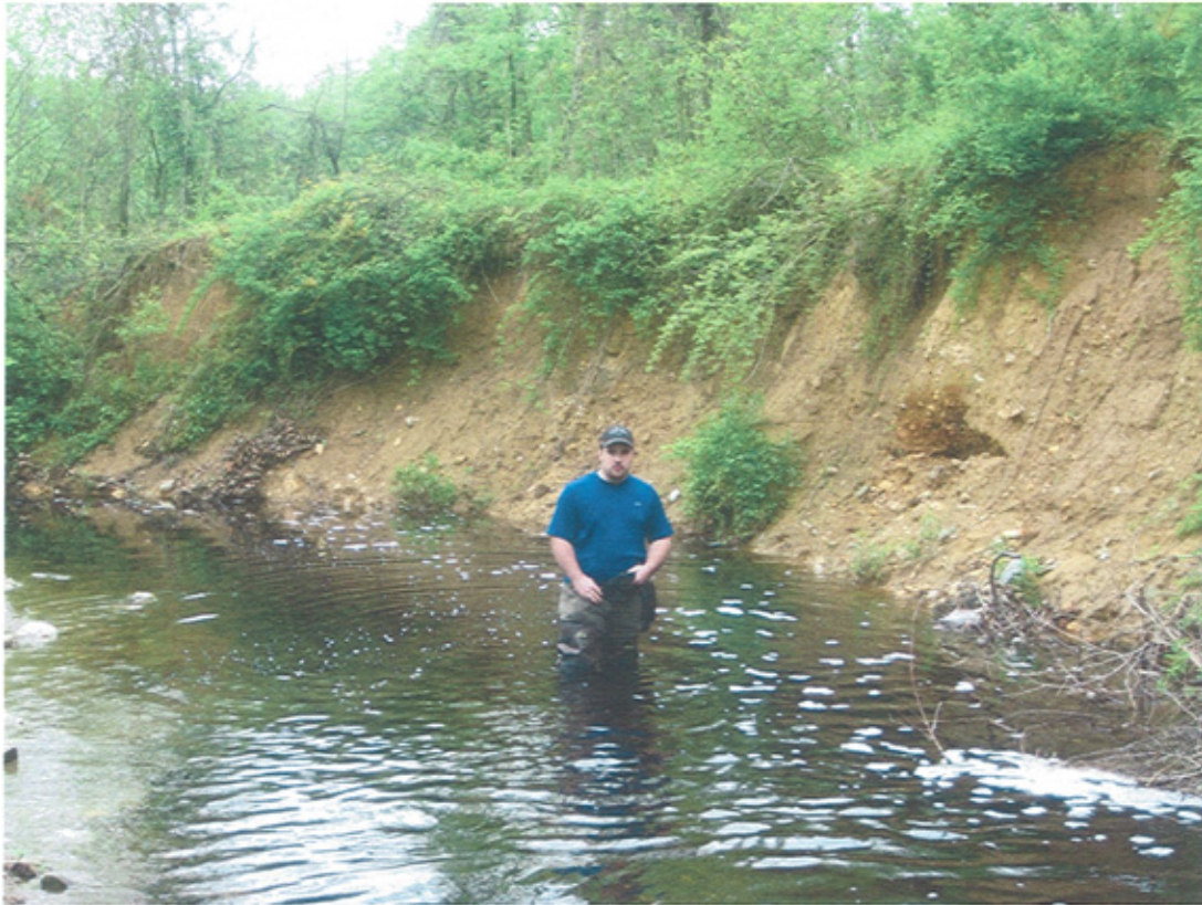
Eroding stream bank.
