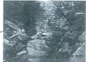
RELOCATE LARGE ROCKS FROM NARROW PORTION OF CHANNEL TO TOE OF ERODED SLOPES AS FIELD DIRECTED.
