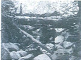
REMOVE EXISTING BRUSH AND LOG CLOG, GROCERY CART AND OTHER ASSORTED TRASH AND DEBRIS FROM STREAM CHANNEL
