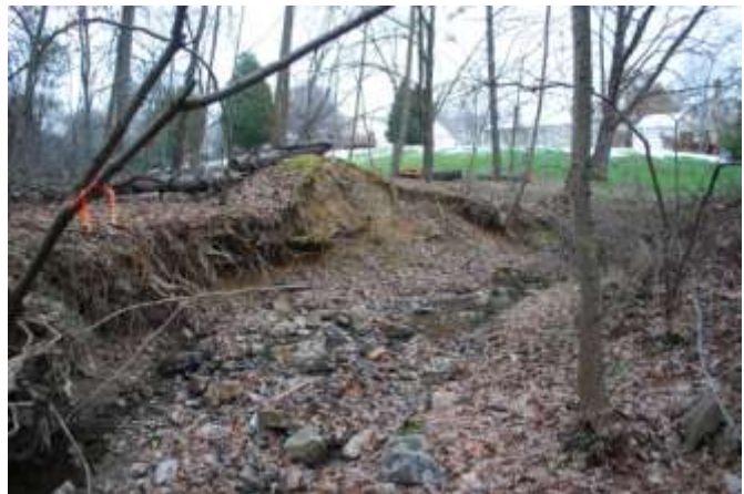
Section of eroded stream channel
