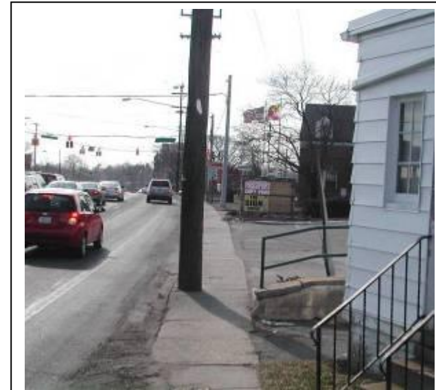
Existing Condition: This pedestrian path is unsafe due to obstructions and its proximity to high speed vehicular traffic.
