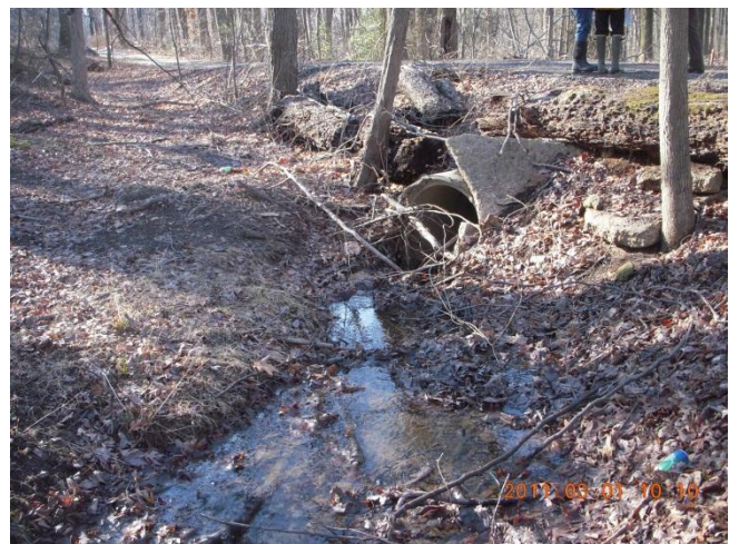
Failing Driveway Culvert
