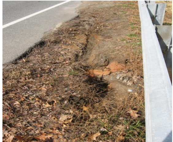
Figure 5: Erosion from roadside rutting
