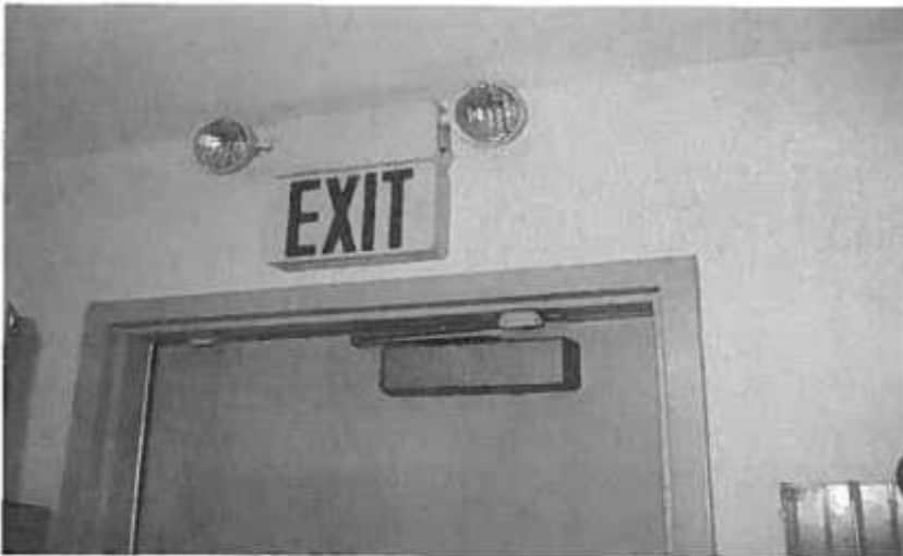
PHOTOGRAPH 4: Exit Sign Malfunctioning at Adult Education Center
