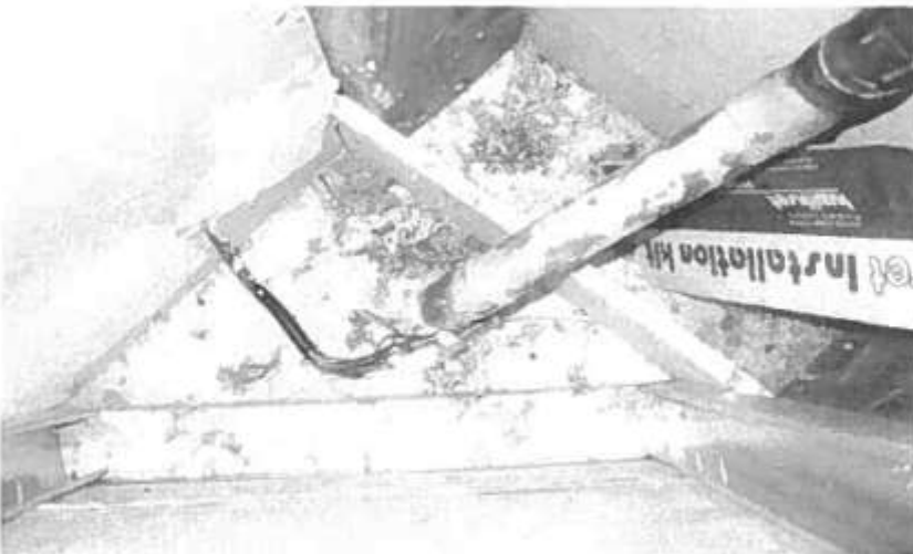
PHOTOGRAPH 3: Disconnected Ground Wire to be Reconnected
