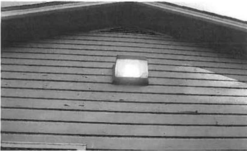
PHOTOGRAPH 1: Paint is Deteriorated and Peeling from Exterior
