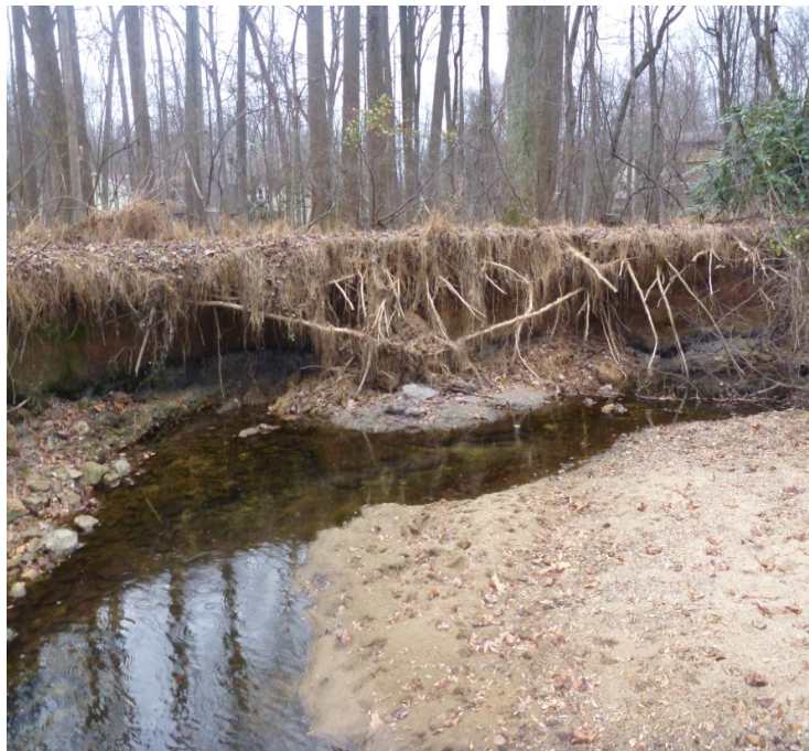
Steep, actively eroding bank along Hollywood Branch
