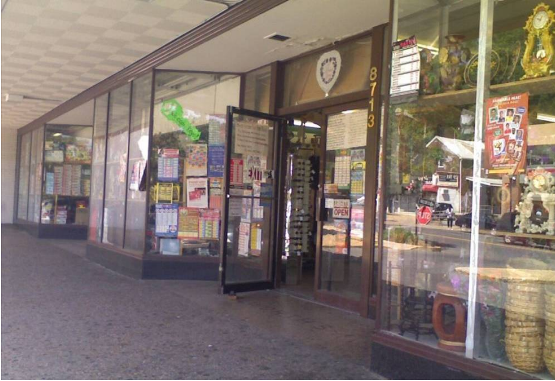
The Woolworth storefront (8713) has a high level of integrity with original window walls, black marble base, and ribbed metal cornice. Terrazzo Floor (below). (Clare Lise Kelly, M-NCPPC, 6-2010)
