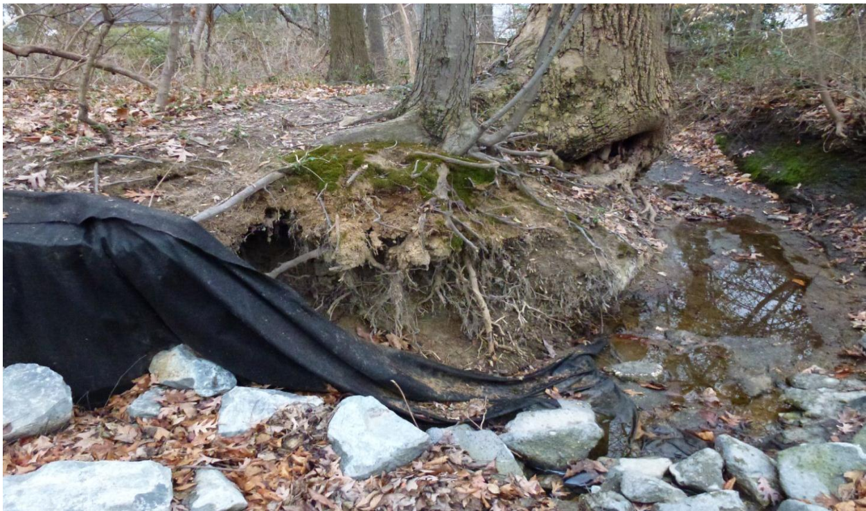
Apparent lack of mitigation measures for critically damaged root zones
