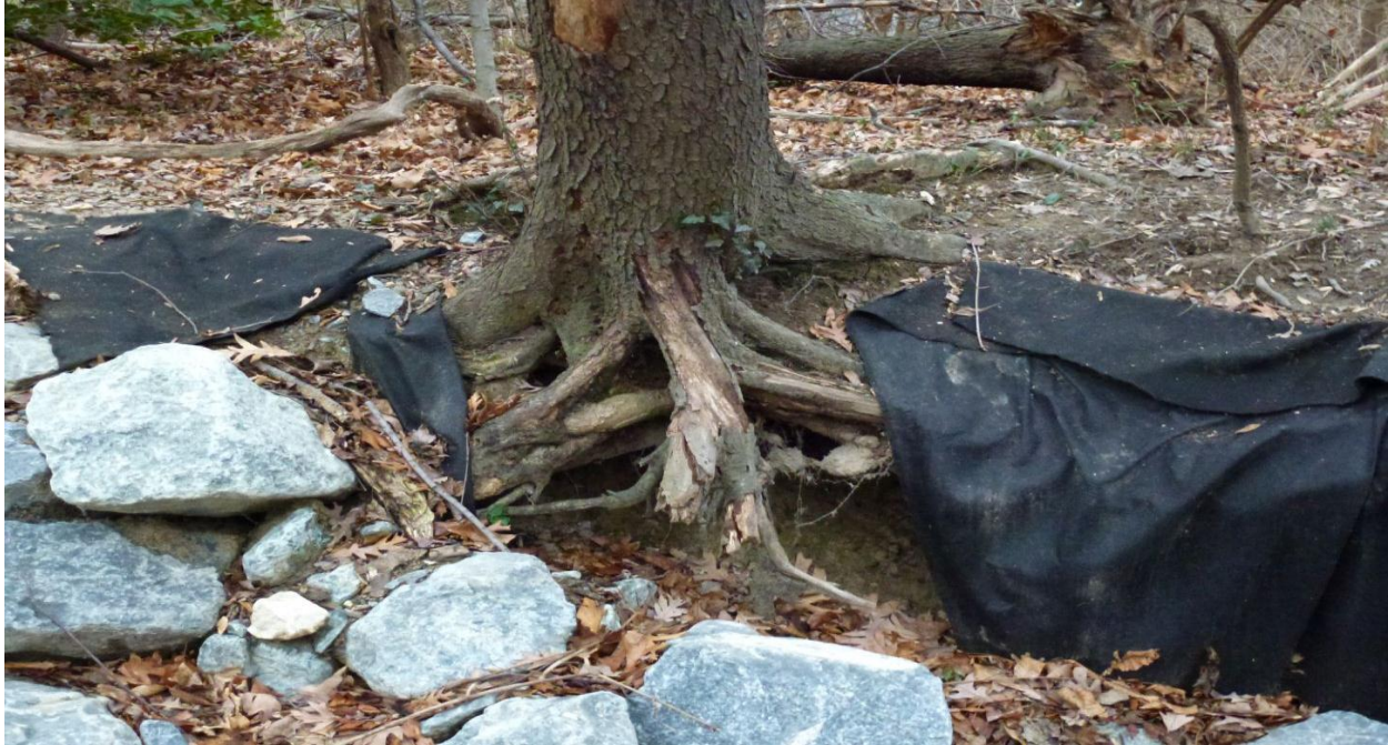
Sediment control failure – silt fence
