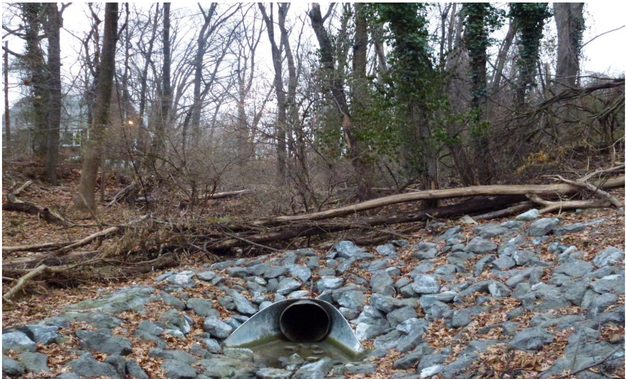
Upstream connection to Costco detention tanks
