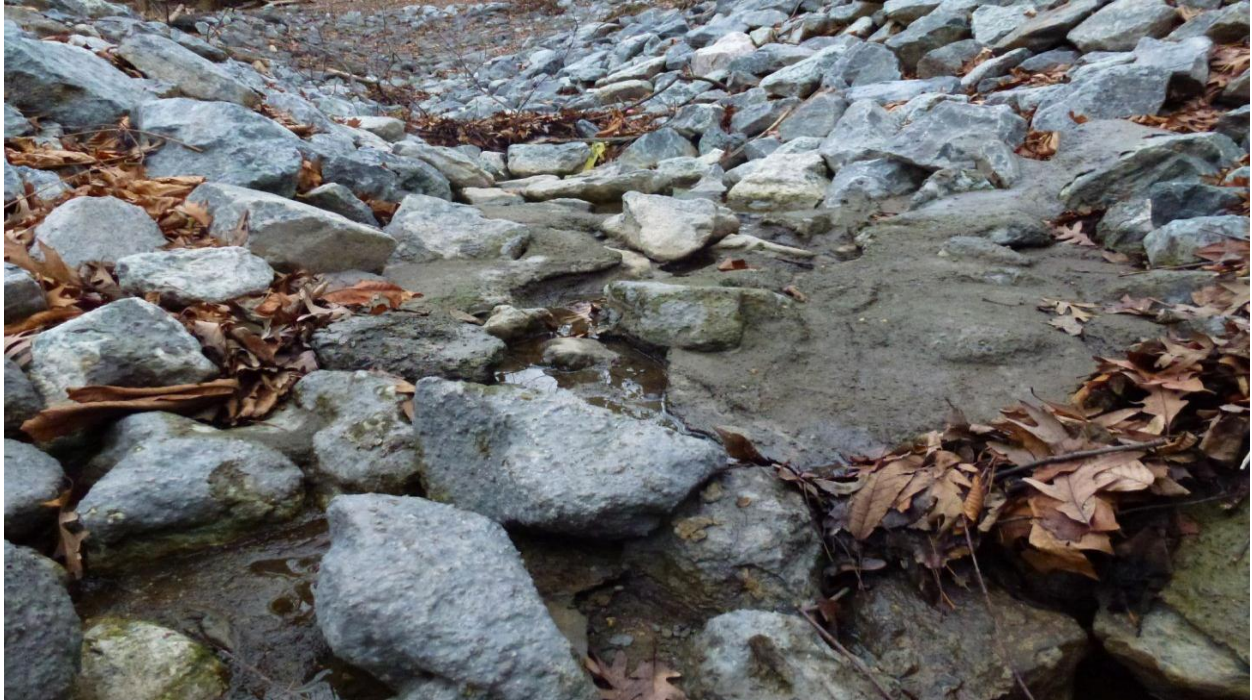
Riprap at downstream end is starting to dislodge
