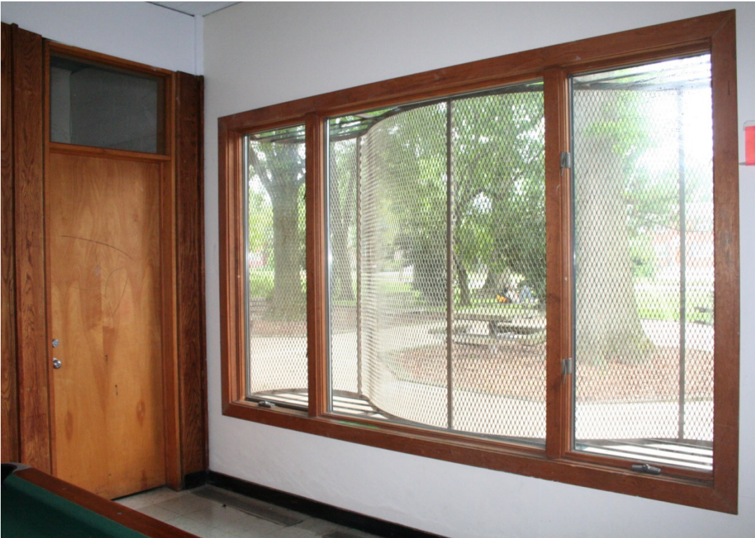
FIGURE 24: Fixed windows and flanking casement sash have replacement double pane glass in original wood frames. Metal screens were installed on the exterior as a safety measure. (Clare Lise Kelly, Jun 2013)
