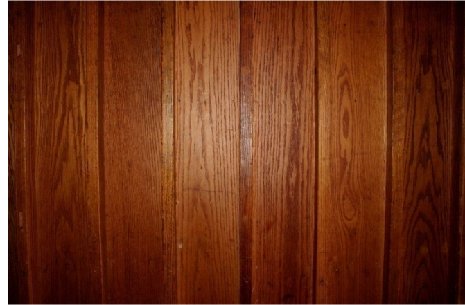
D: Wall paneling in the snack room
