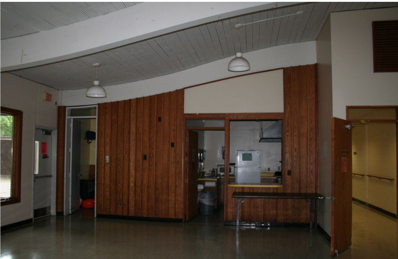
FIGURE 20: Game Room, North wall, current view, with double doors at far right. The interior retains a high level of integrity in design and materials. (Clare Lise Kelly, June 2013)
