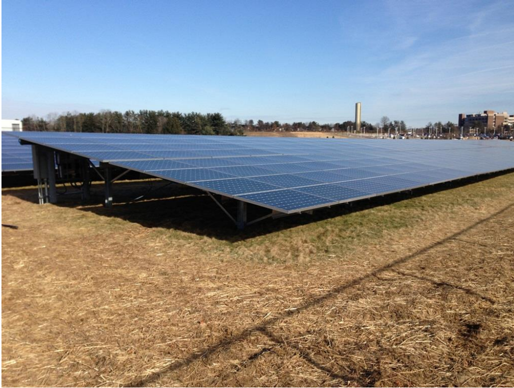
Solar Panels: Ground-mounted Structures
