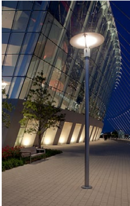
7. Site Lighting for Security
