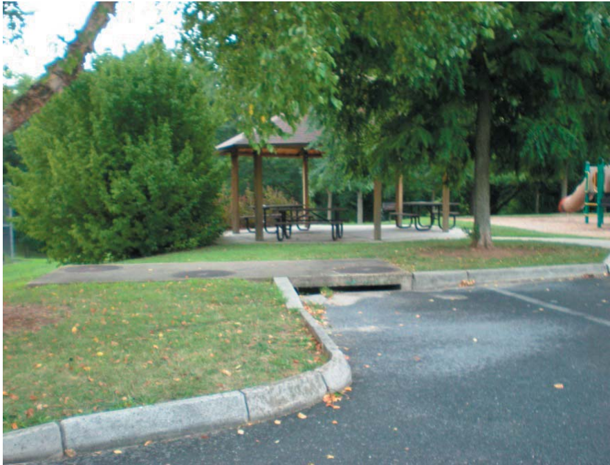
Main Parking Lot Stormwater Vault
