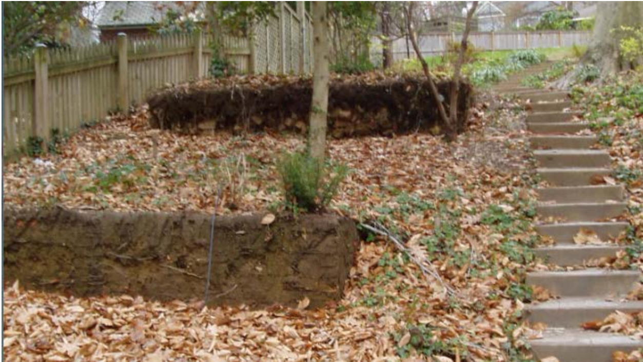
December 2014 photo of exposed vertical soils/rubble remaining after demolition of retaining walls
