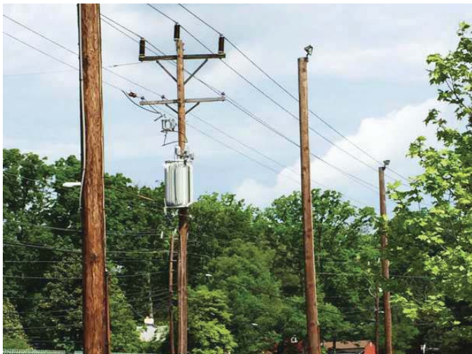
ABOVE GROUND UTILITIES
