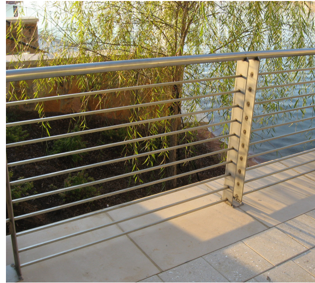
Metal guard rail
