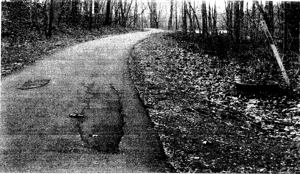
Photo – 3. Pavement Failure
