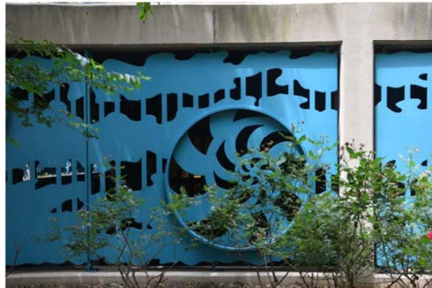
Typical large Garden Screen panel. Note the lack of top and bottom framing which could cause flexing and damage during transport if not stiffened with framing bolted-on to the existing brackets.
